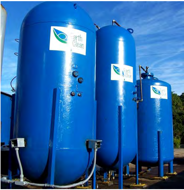
Daphne Utilities Biodiesel Plant
